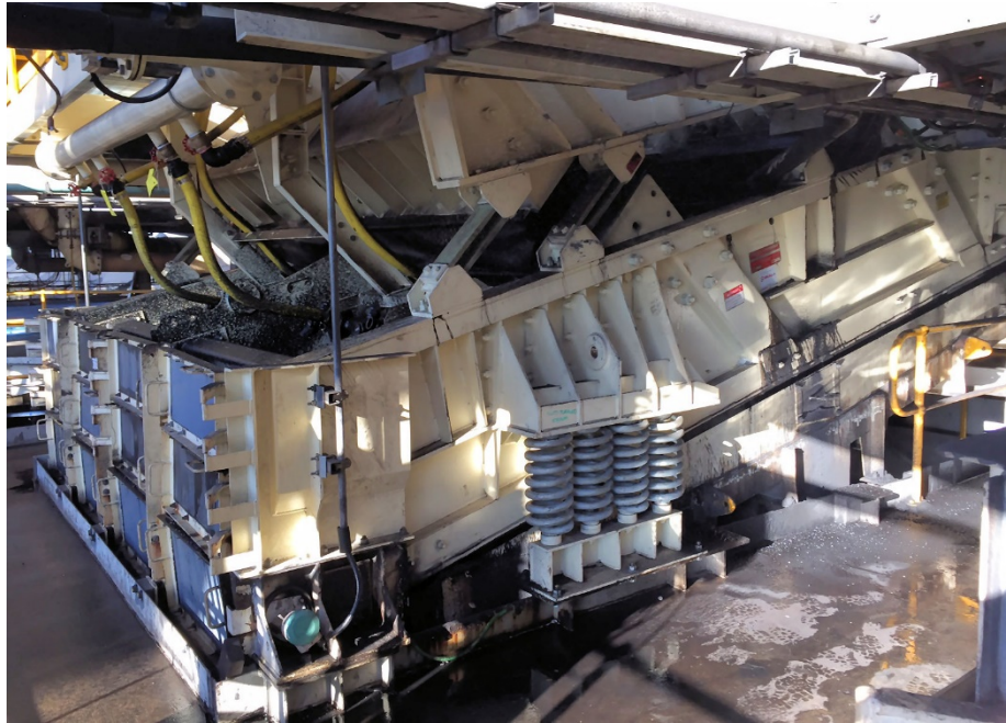
Fig 10 As Installed two mass 3.6 m x 6.1 m 800 t/h rejects drain and rinse screen
